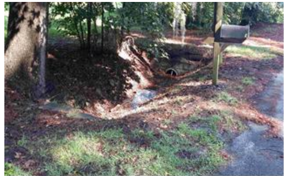
Single family residential lot with large drainage ditch in front yard
