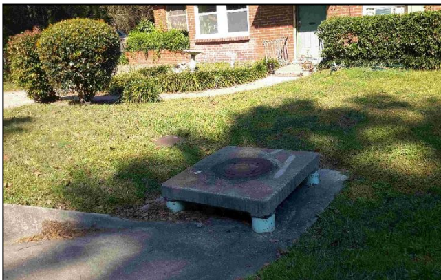
Stormwater drain in front yard
