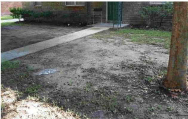
Signs of flooding in front of multi-family residential property
