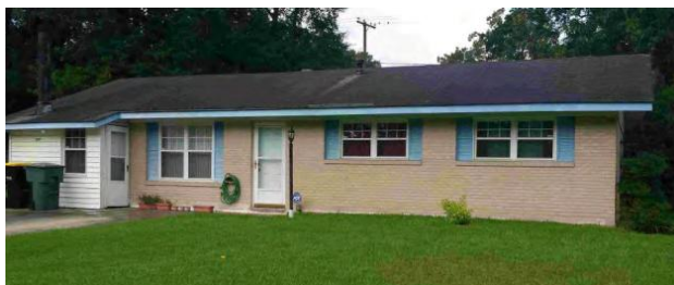
Slab-on-grade house with no gutters
