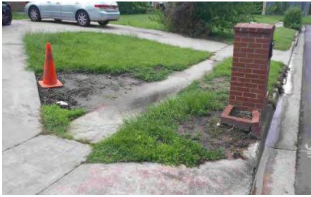
Front yard with flooding damage
