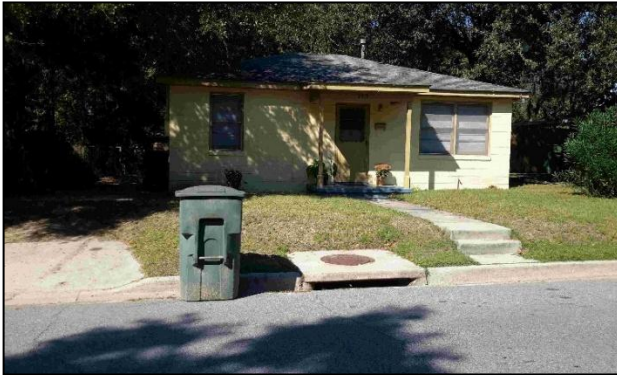
Slab-on-grade house lacking gutters and has a drainage inlet in front yard
