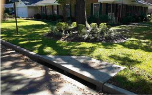
Slab-on-grade house with no gutters and a storm drain on the front corner of the property
