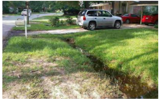
Single-family residential lot with flooded culvert in front yard
