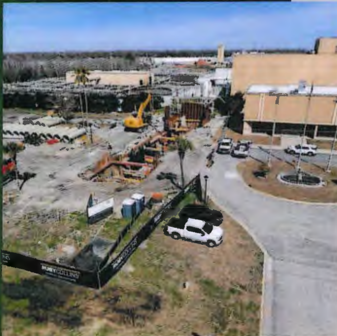
Aerial of twin 60 Installation
