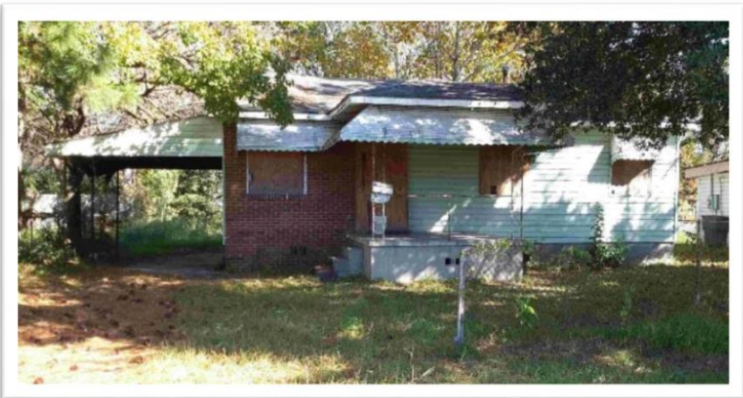
Below: One of several homes listed in the City of Savannah's Local Flooded Structures Database.
