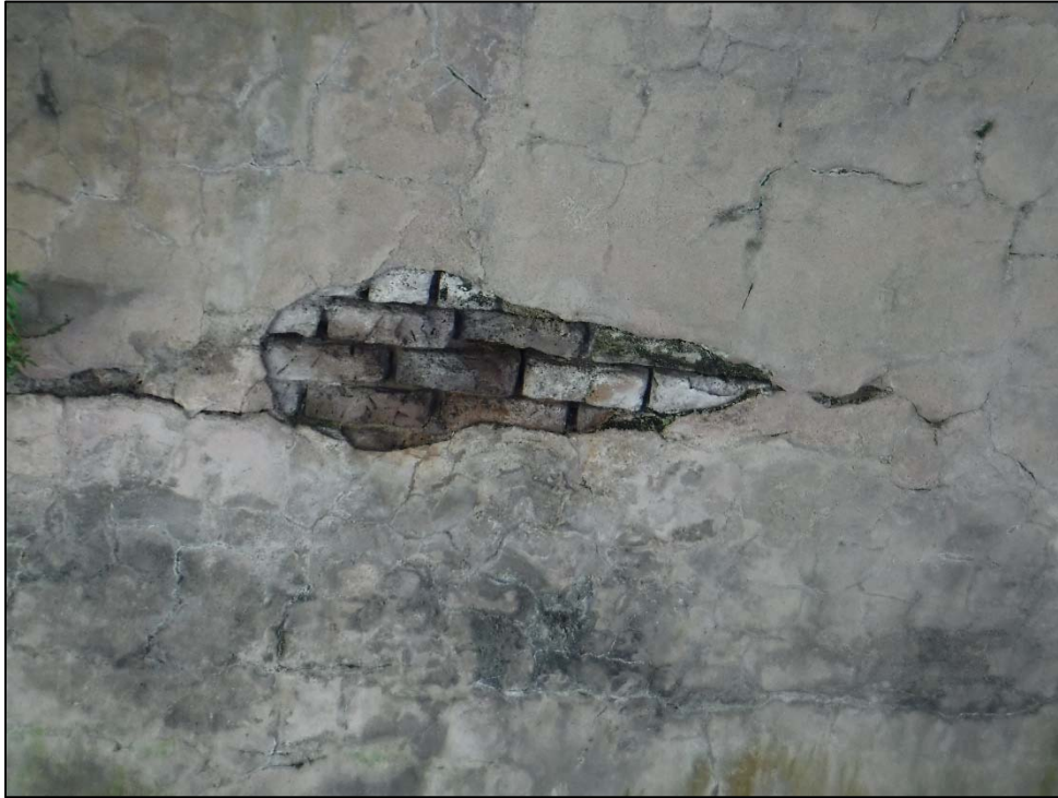
Photograph 81 – Spalled Mortar in Arch 2
