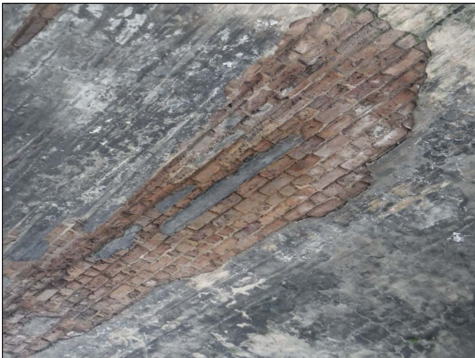
Photograph 84 – Spalled Mortar in Arch 3
