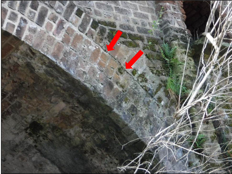
Photograph 27 – Crack in Masonry Arch Ring in Arch 4
