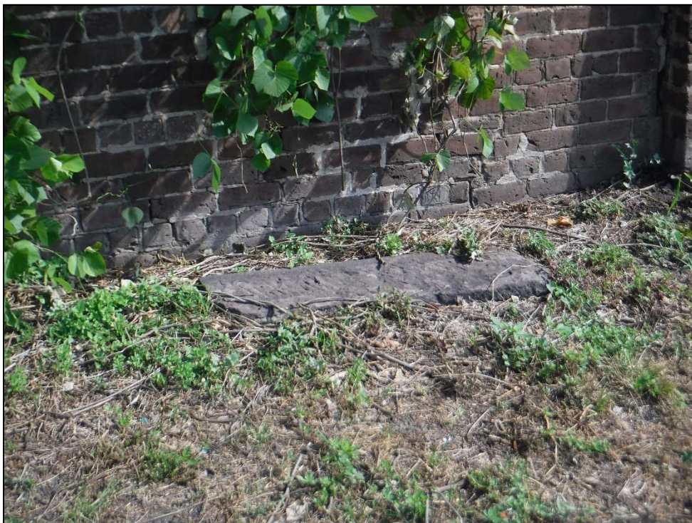
Photograph 104 – Dislodged Coping Piece at Southwest Wingwall
