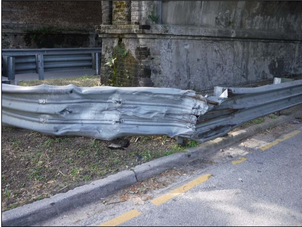
Photograph 41 – Guard Rail Impact Damage at Pier 3
