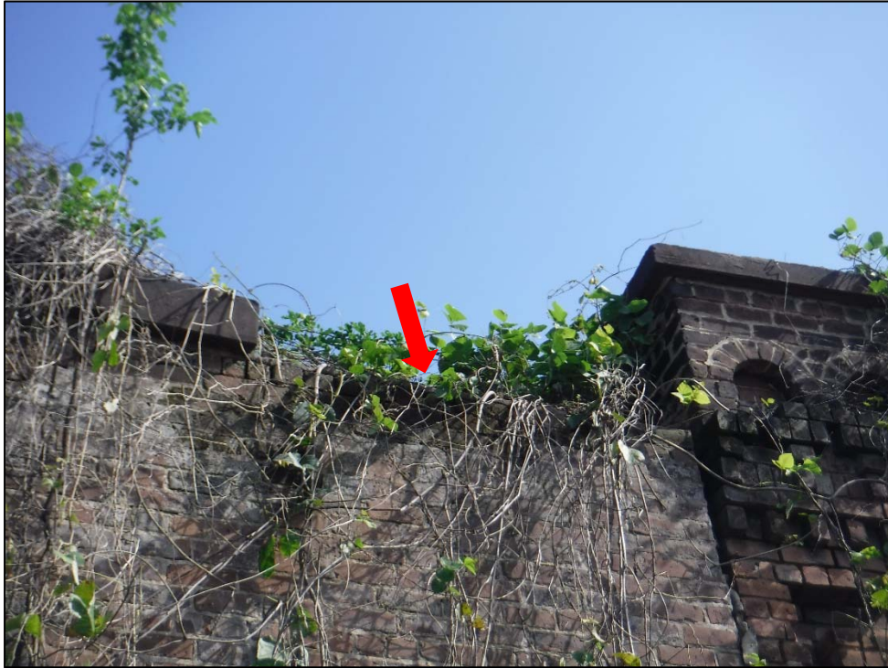
Photograph 103 – Dislodged Coping Piece at Southwest Wingwall
