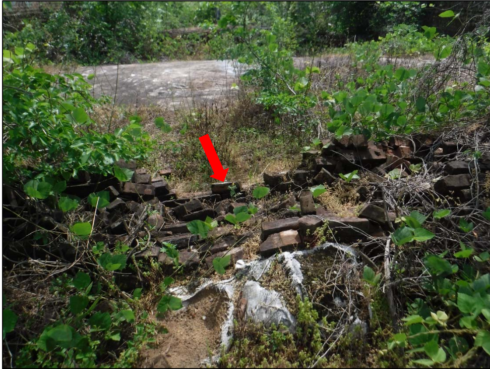
Photograph 17 – Collapsed Portions of Open Drainage Arches
