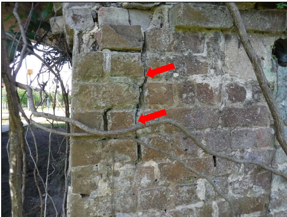
Photograph 28 – Crack with Damaged Bricks at Pier 1
