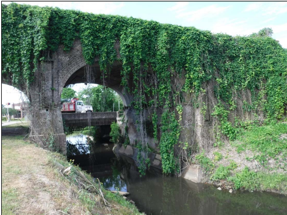
Photograph 36 – Vegetation Growth Throughout North Elevation
