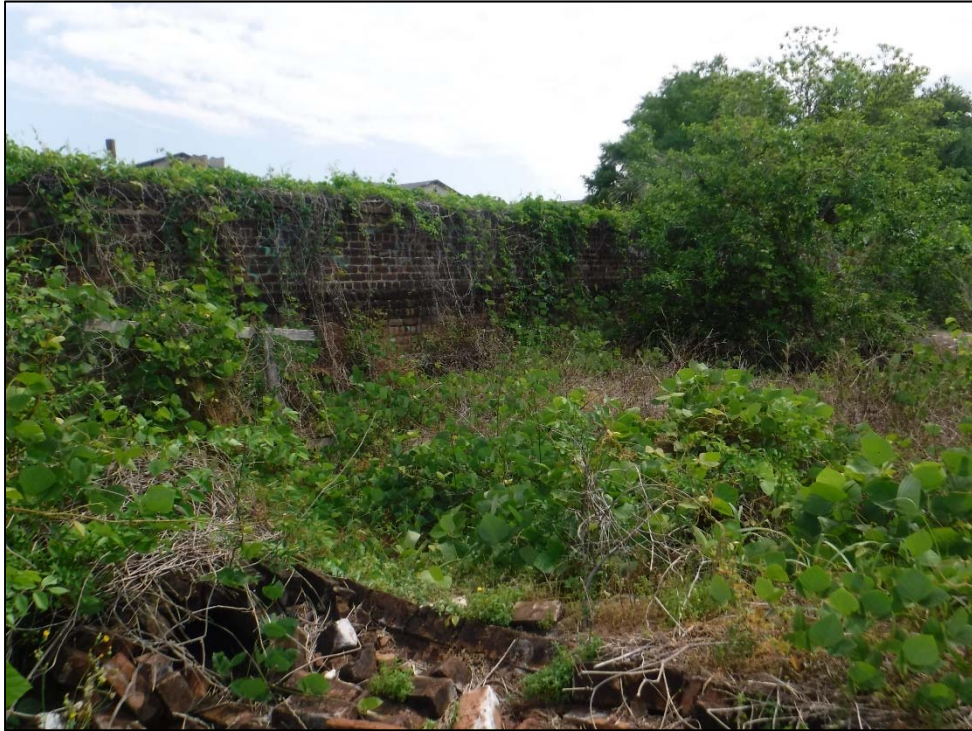
Photograph 21 – Heavy Vegetation Growth atop Viaduct
