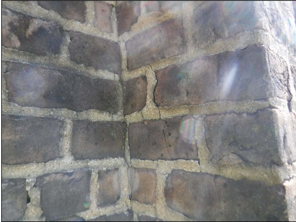
Photograph 47 – Crack with Damaged Bricks
