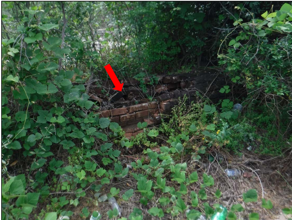
Photograph 18 – Collapsed Portions of Open Drainage Arches
