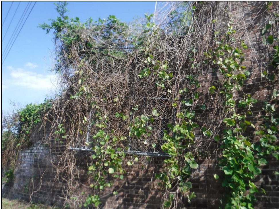
Photograph 102 – Fallen Fence in Vegetation Growth at Southwest Wingwall
