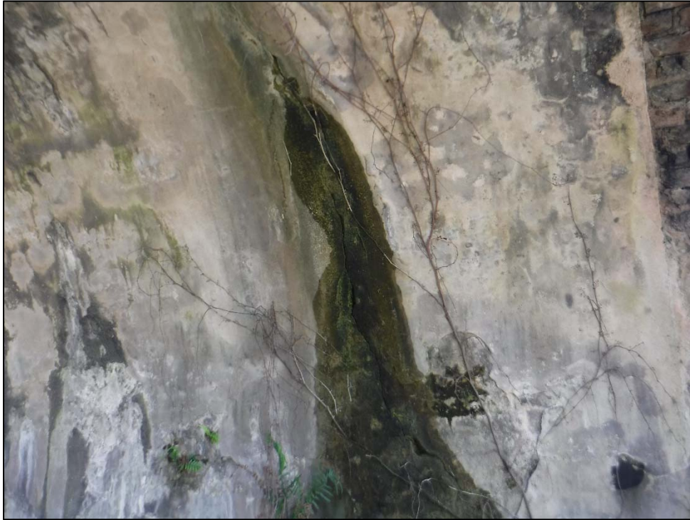
Photograph 79 – Active Water Seepage Through Mortar Cracks in Arch 2
