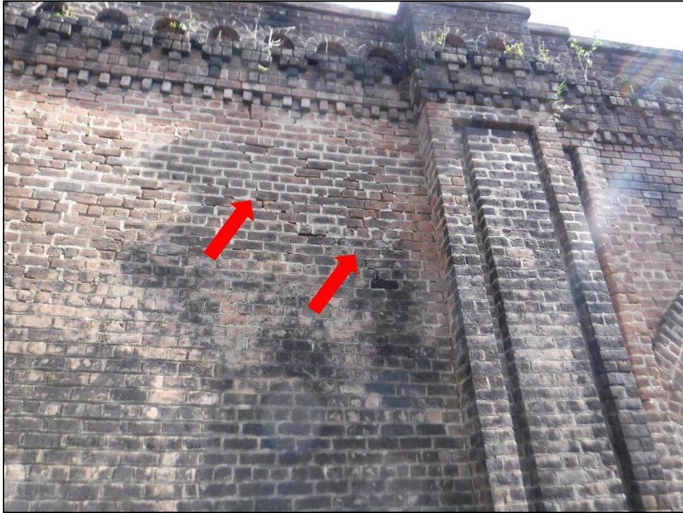
Photograph 45 – Crack with Damaged Bricks
