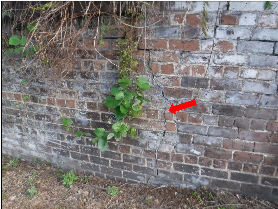
Photograph 96 – Vertical Crack with Damaged Brick in Southwest Wingwall
