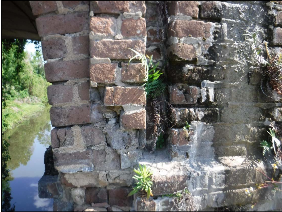
Photograph 53 – Damaged and Cracked or Missing Bricks in Arch 1
