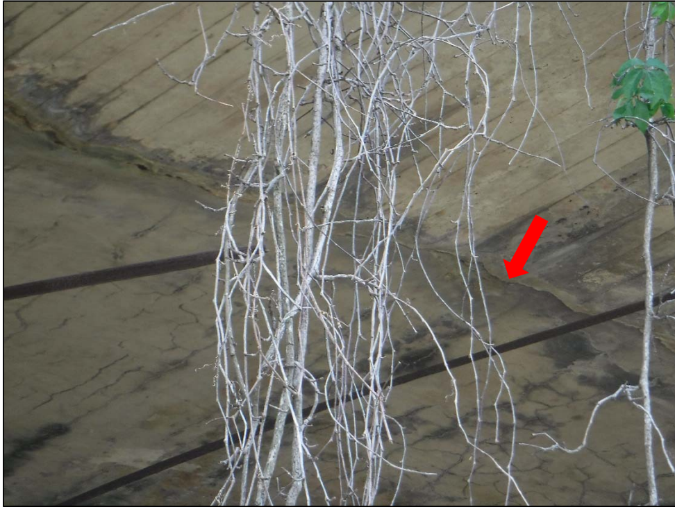
Photograph 73 – Crack with Spalled Mortar in Arch 1
