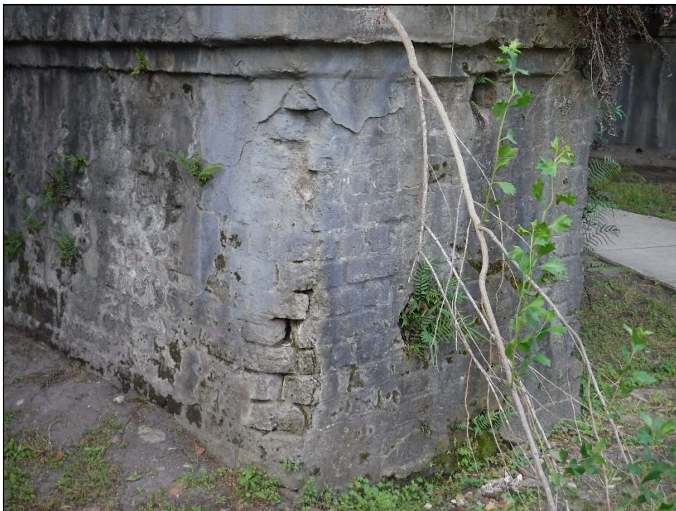
Photograph 32 – Deteriorated Previous Repair and Brick Masonry in Weep Drains
