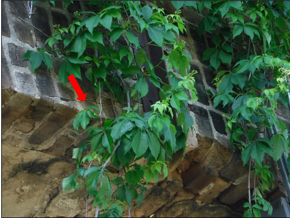
Photograph 31 – Crack with Damaged/Cracked Bricks in Arch 2
