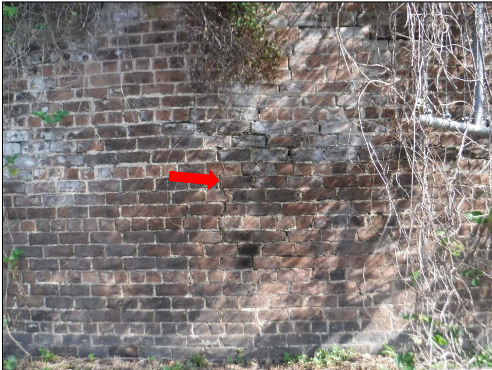
Photograph 94 – Vertical Crack with Damaged Brick in Southwest Wingwall
