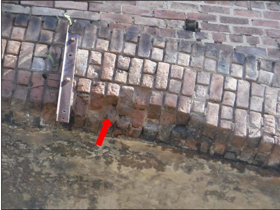
Photograph 57 – Damaged/Missing Brick in Arches
