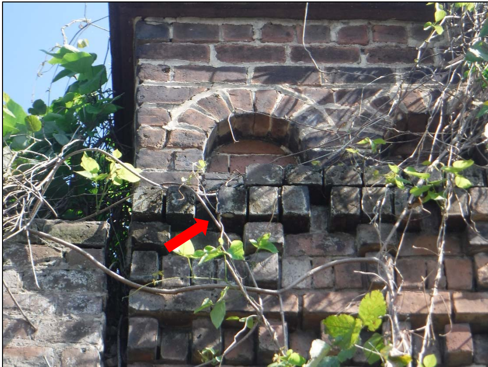
Photograph 62 – Missing Bricks in Viaduct
