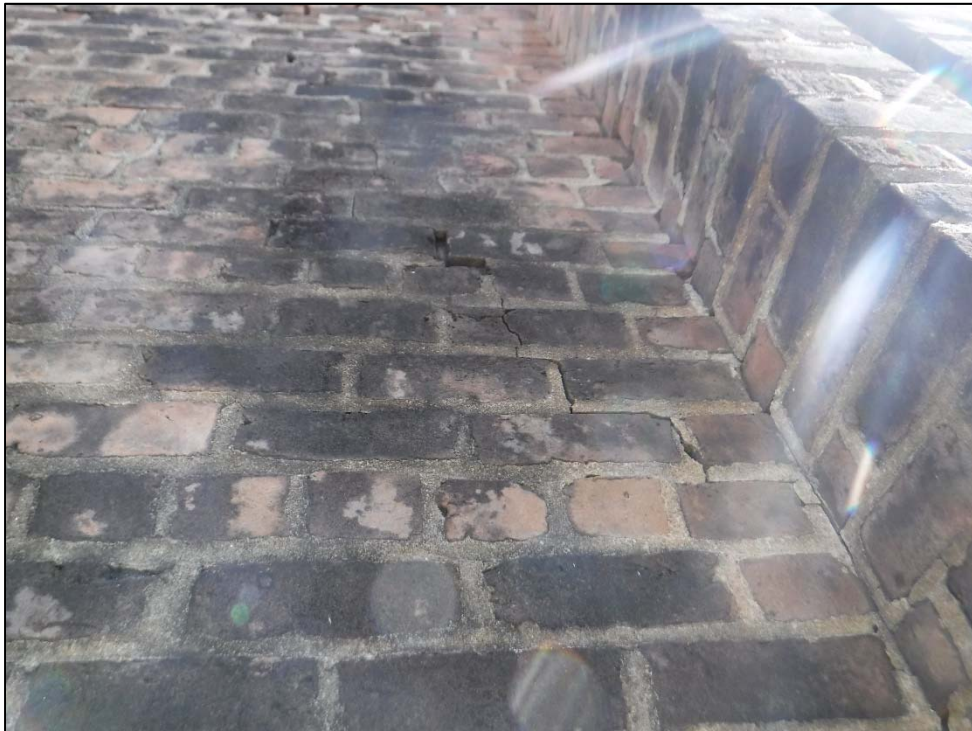
Photograph 46 – Crack with Damaged Bricks
