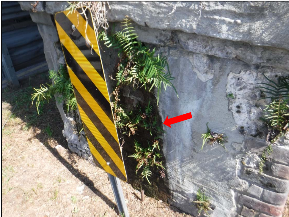
Photograph 58 – Vegetation Growth and Staining
