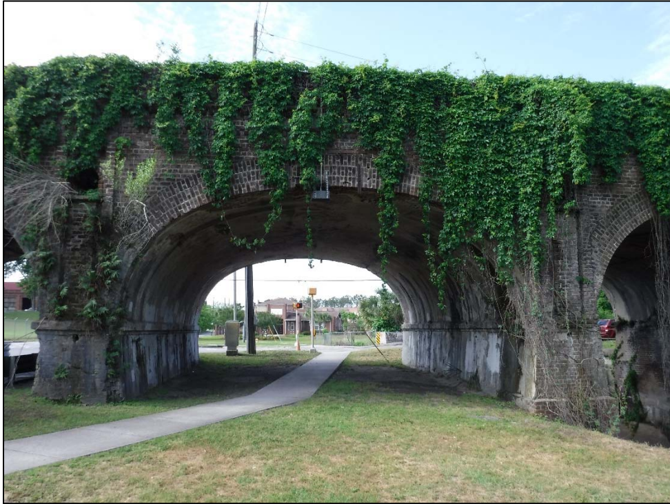
Photograph 37 – Vegetation Growth Throughout North Elevation
