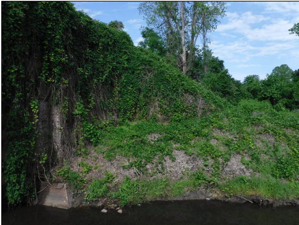
Photograph 90 – Vegetation Growth at Northwest Wingwall
