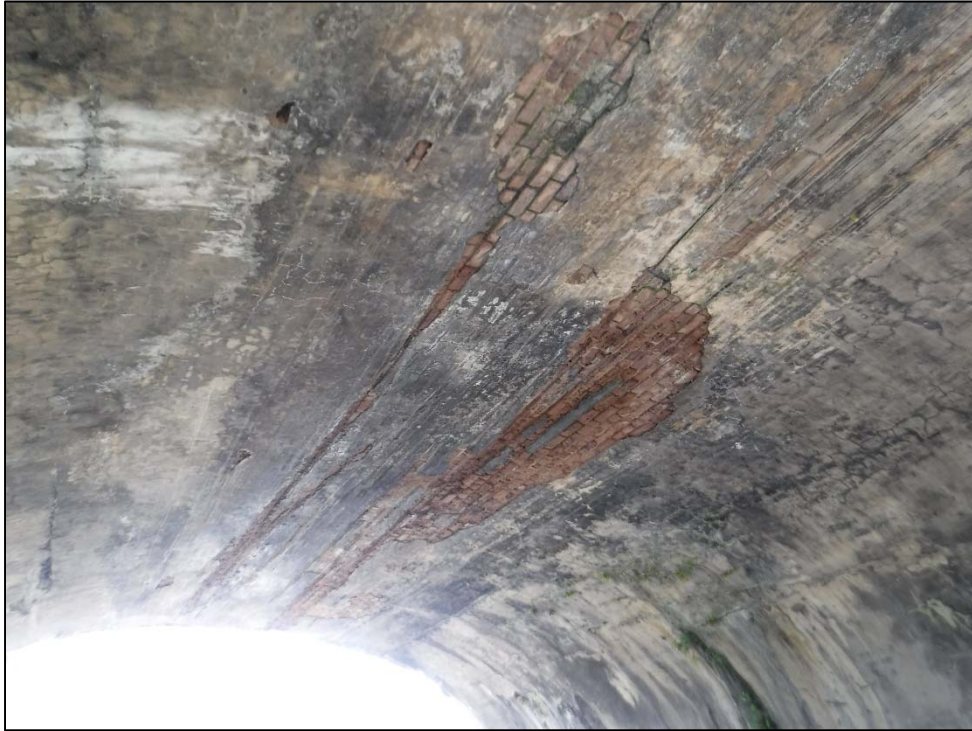
Photograph 83 – Spalled Mortar in Arch 3
