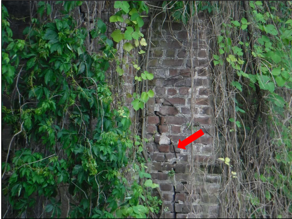
Photograph 71 – Crack with Spalled Mortar in Arch 1
