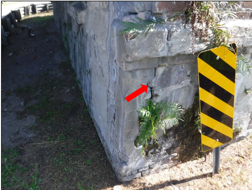
Photograph 54 – Crack with Differential Displacement at Pier 3
