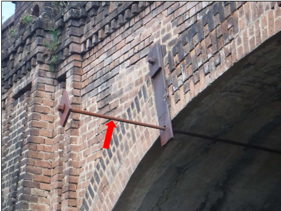
Photograph 76 – Failed Post-Tensioning Tie Rods at Arch 1
