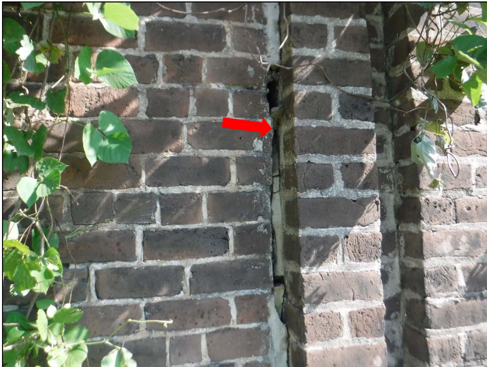
Photograph 98 – Mortar Loss Along Construction Joint in Southwest Wingwall
