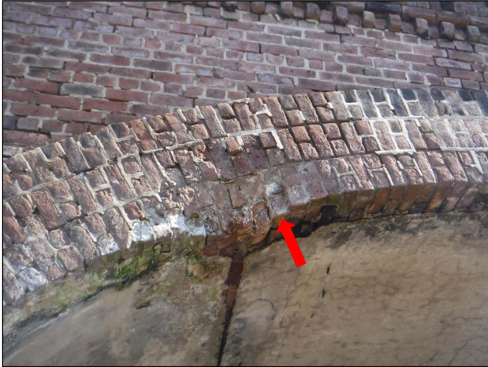
Photograph 55 – Damaged/Missing Brick in Arches
