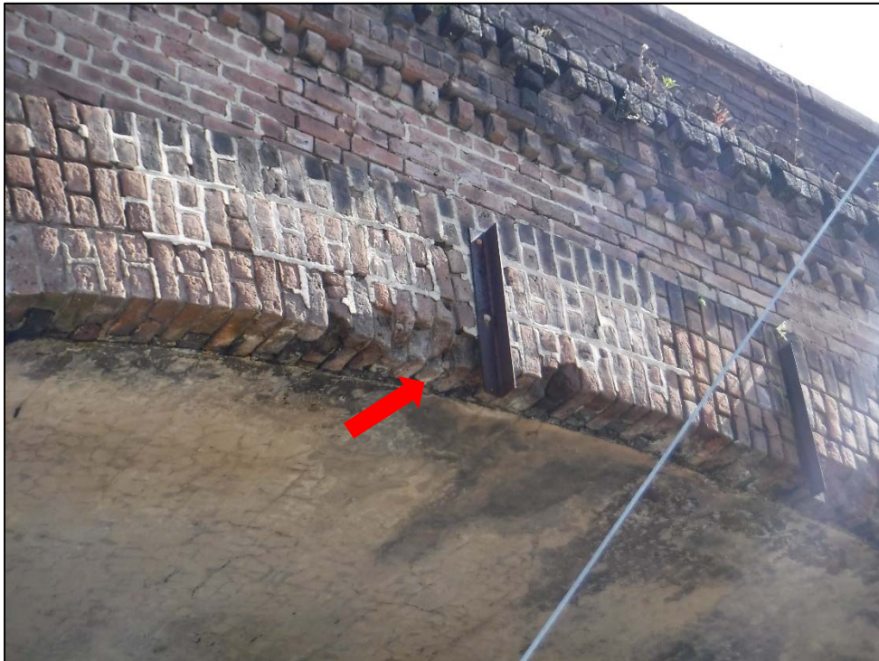
Photograph 56 – Damaged/Missing Brick in Arches
