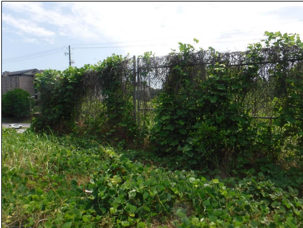
Photograph 24 – Fence with Vegetation Growth Blocking West Approach
