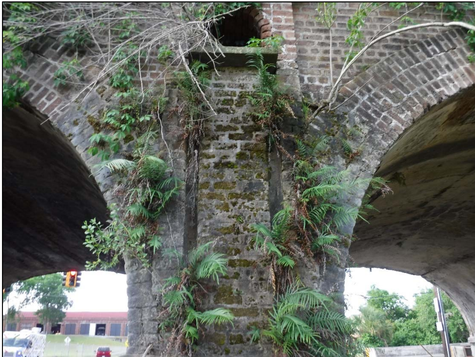
Photograph 38 – Vegetation Growth Throughout North Elevation
