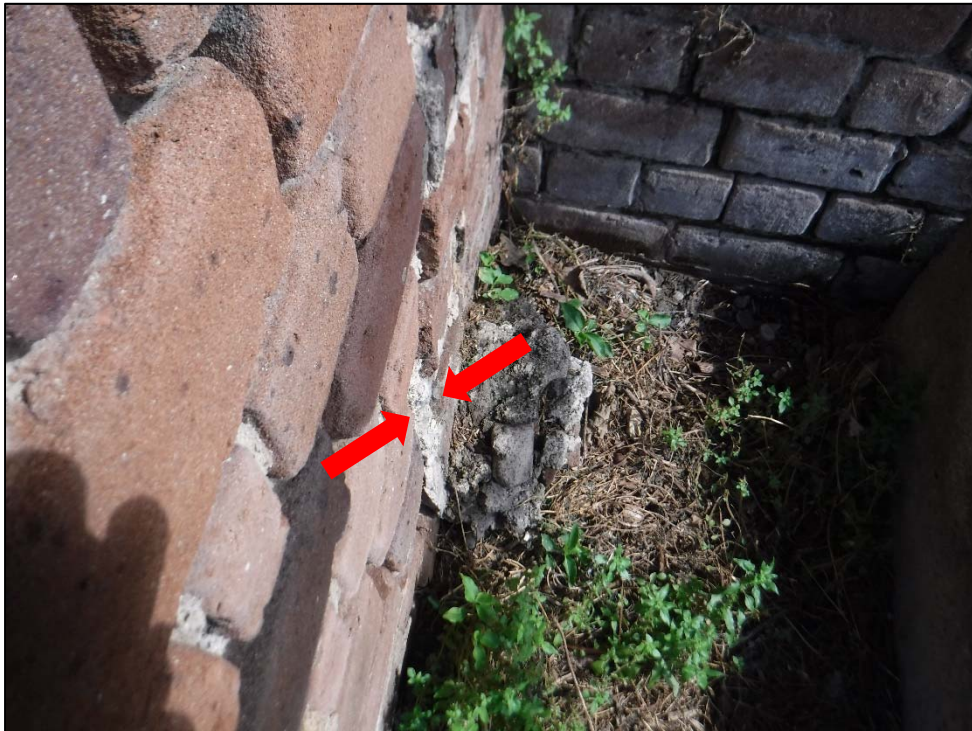
Photograph 52 – Crack with Differential Displacement
