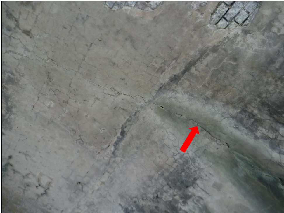
Photograph 78 – Crack Across Underside of Arch 2
