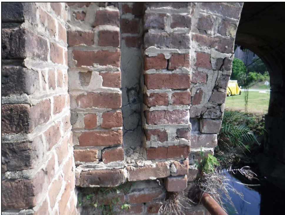
Photograph 50 – Cracked/Spalled Mortar Parging with Missing And Damaged Bricks at Arch 4
