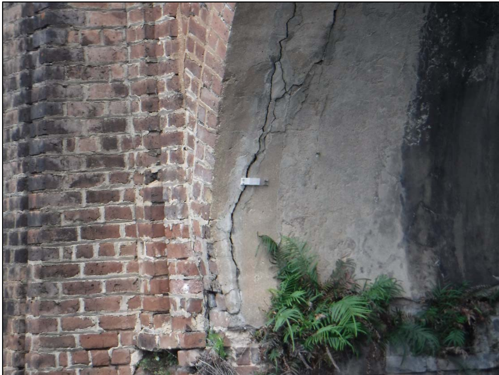
Photograph 70 – Crack Across Underside of Arch 1
