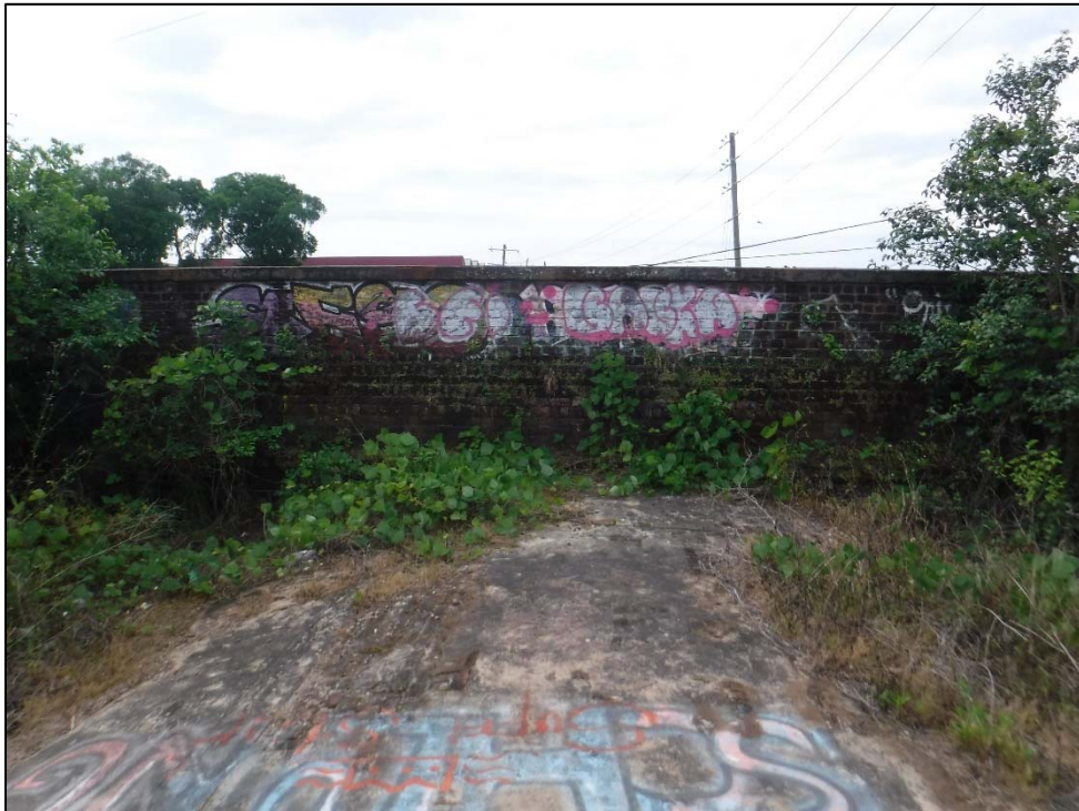
Photograph 22 – Graffiti on Brick Masonry
