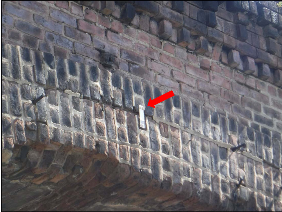
Photograph 65 – Crack Gauge Above Arch 3
