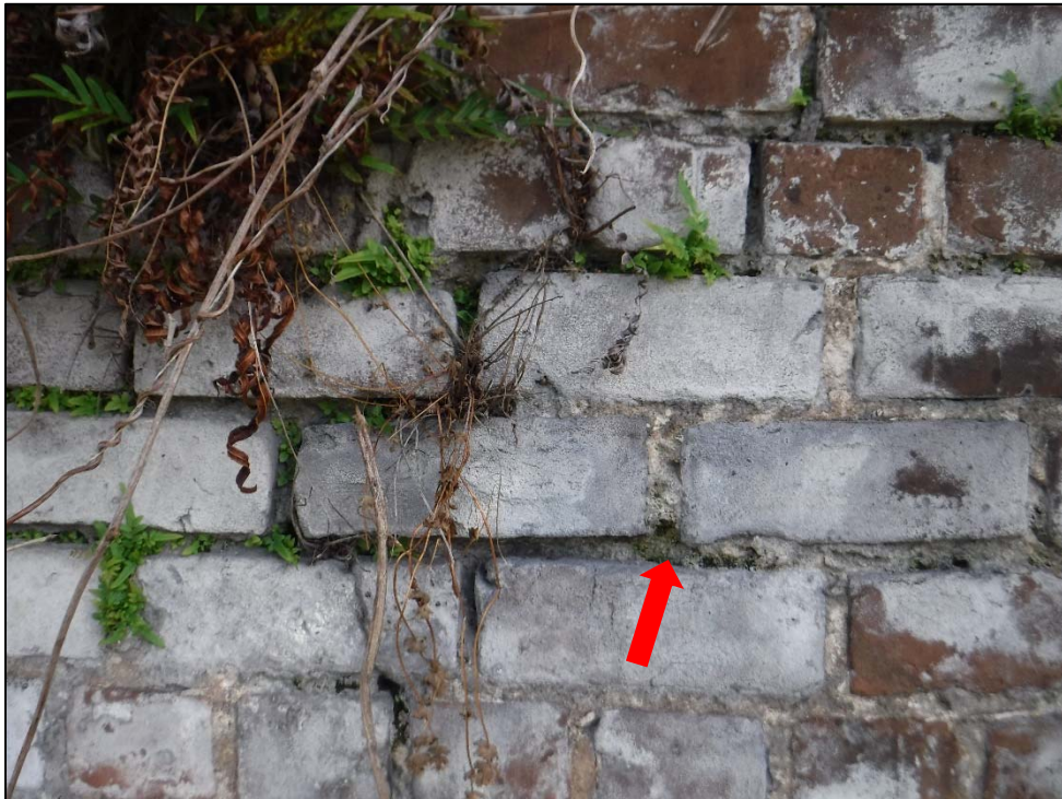
Photograph 100 – Deteriorated/Missing Mortar in Southwest Wingwall
