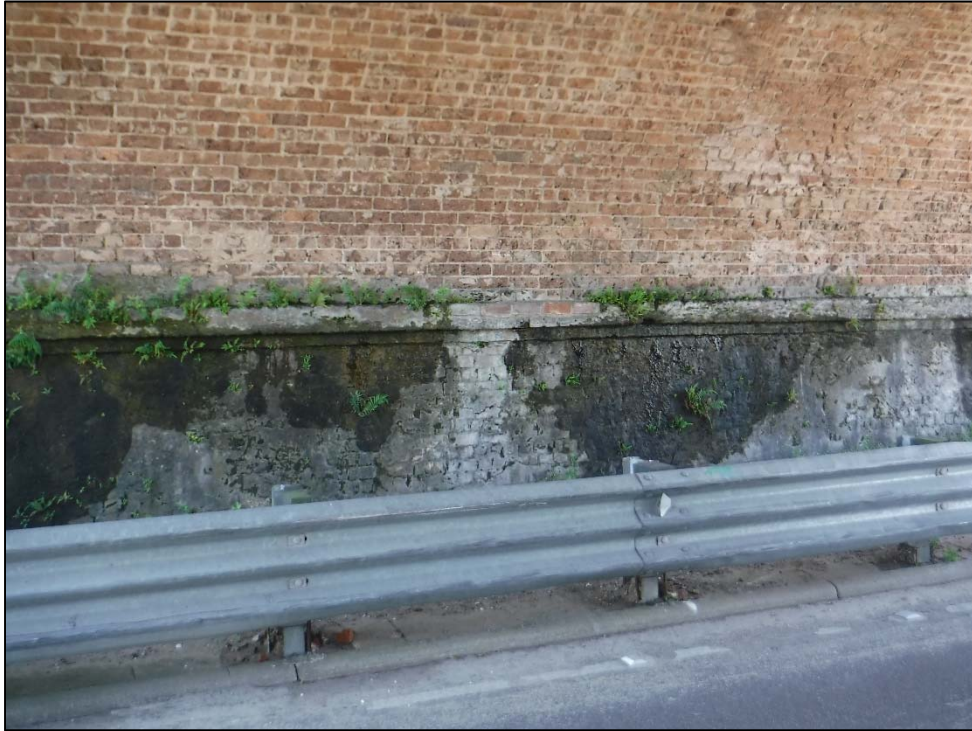
Photograph 87 – Water Staining at Arch 4
