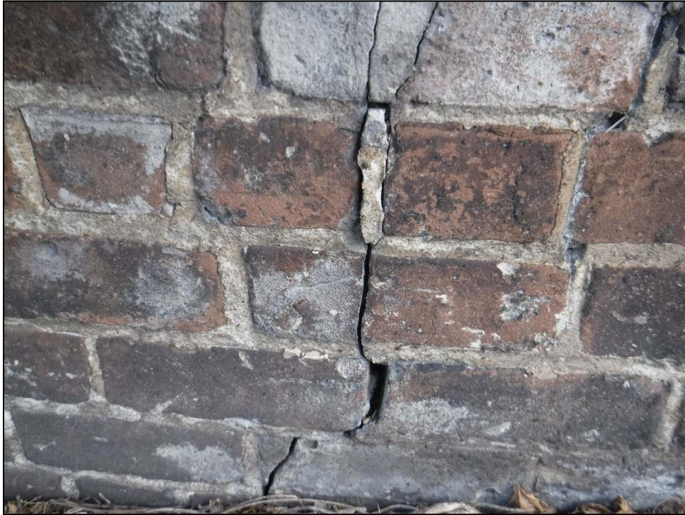
Photograph 97 – Vertical Crack with Damaged Brick in Southwest Wingwall
