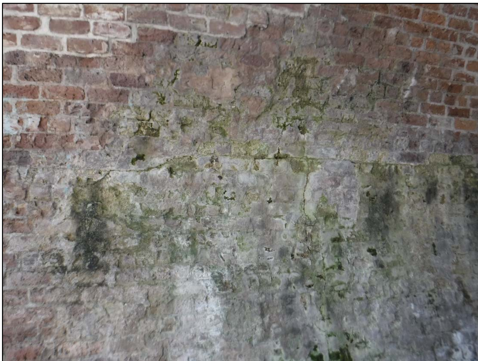
Photograph 86 – Longitudinal and Transverse Cracking in Arch 4
