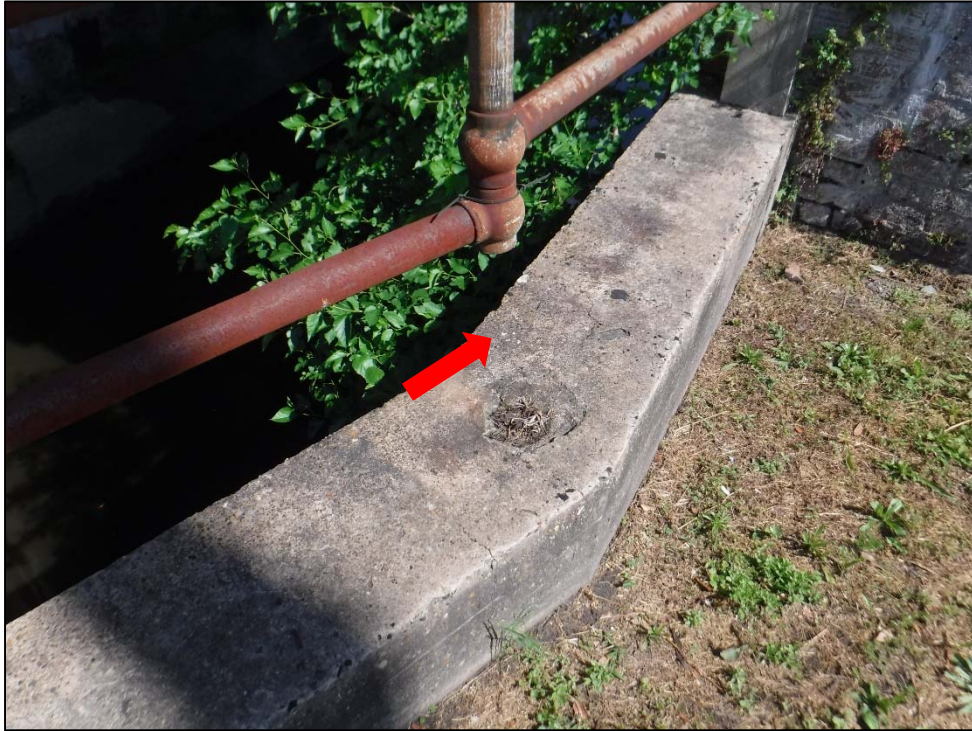
Photograph 67 – Missing Portion of Guardrail at Arch 1
