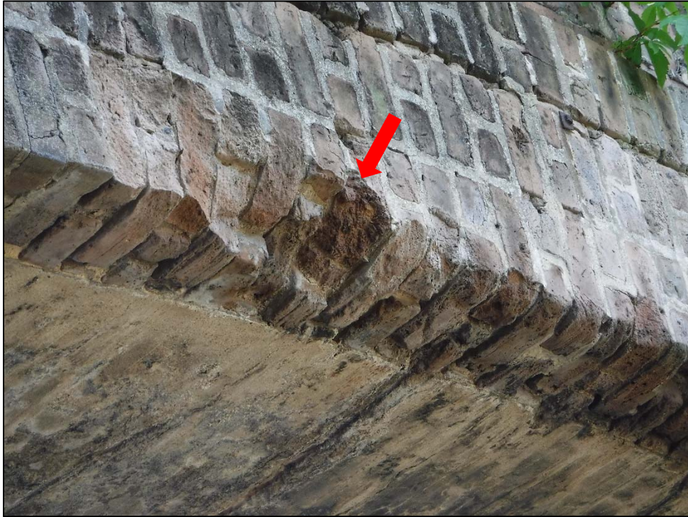
Photograph 33 – Damaged/Missing Brick Masonry in Arches
