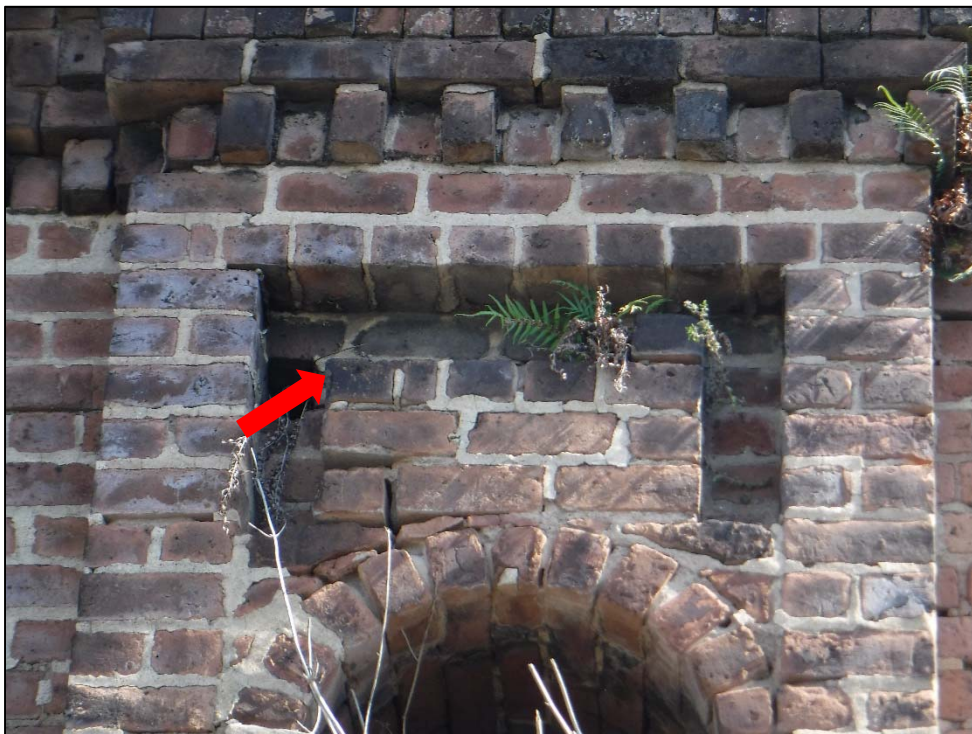
Photograph 64 – Missing Bricks at Pier 2
