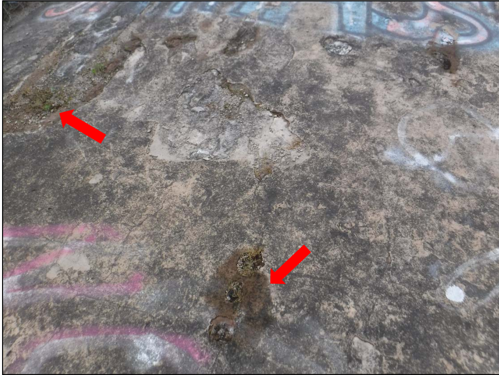
Photograph 15 – Mortar Loss with Exposed Masonry and Vegetation Growth
