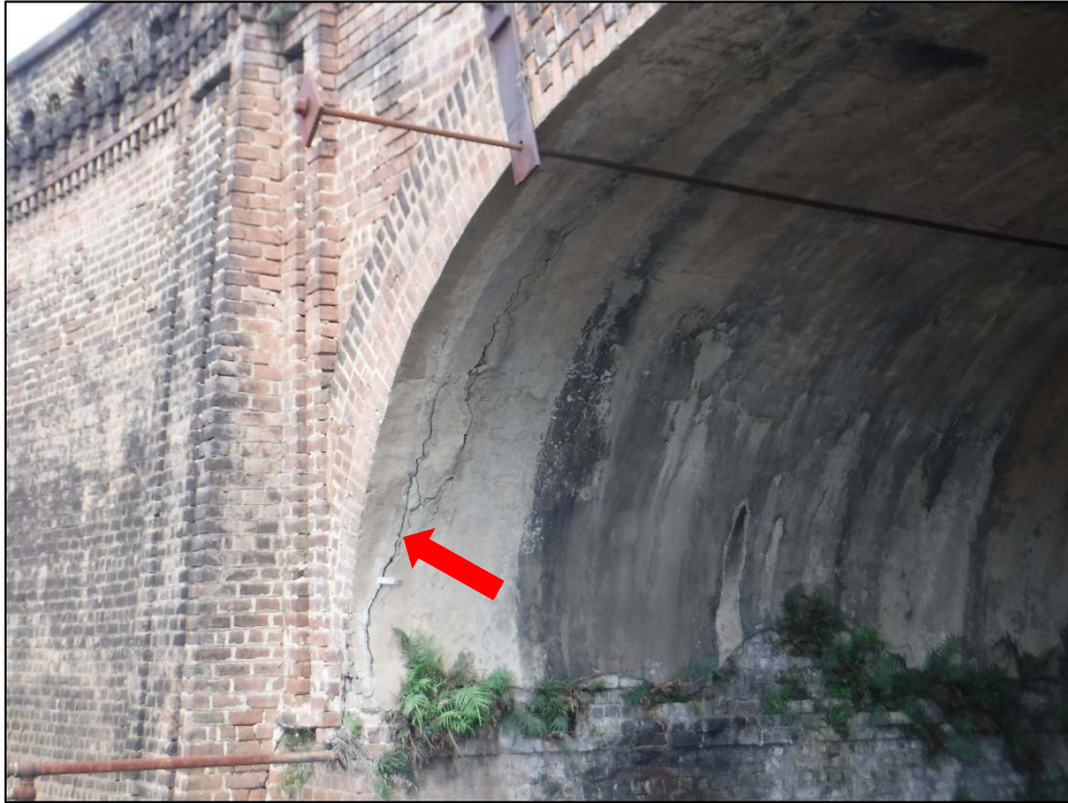
Photograph 69 – Crack Across Underside of Arch 1
