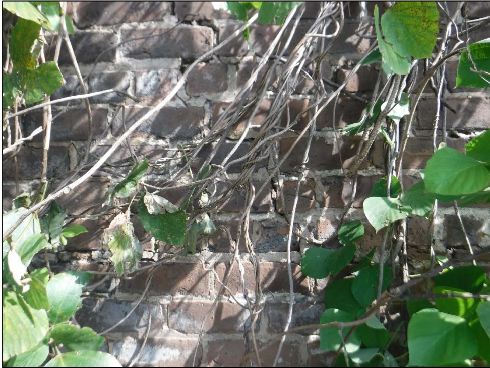
Photograph 91 – Diagonal Crack Obstructed by Vegetation Growth At Southwest Wingwall
