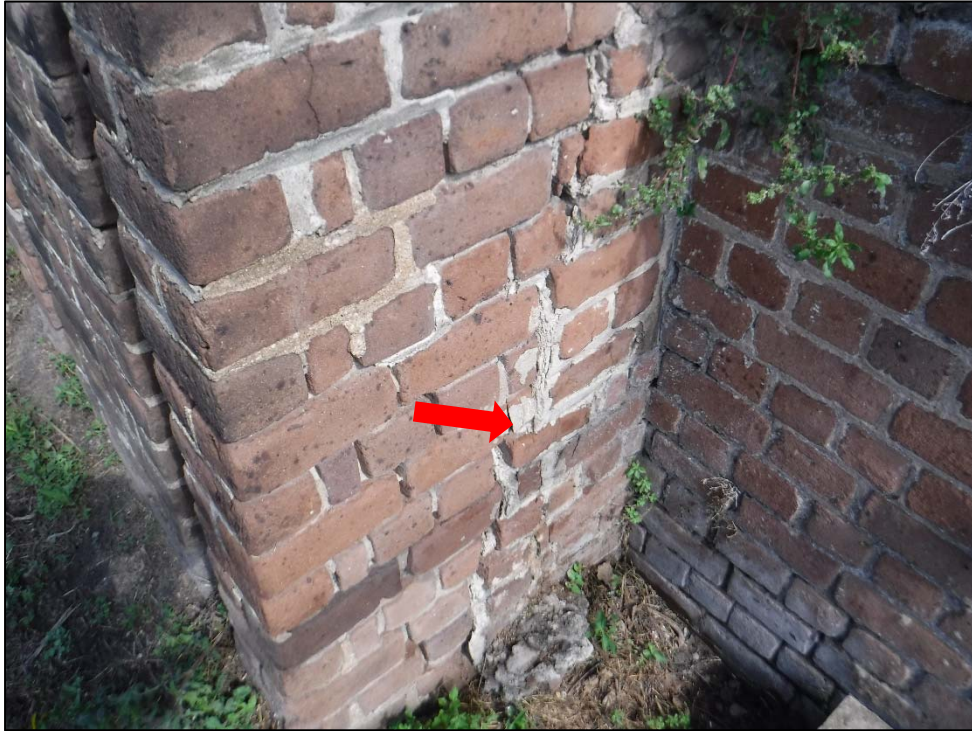
Photograph 51 – Crack with Differential Displacement
