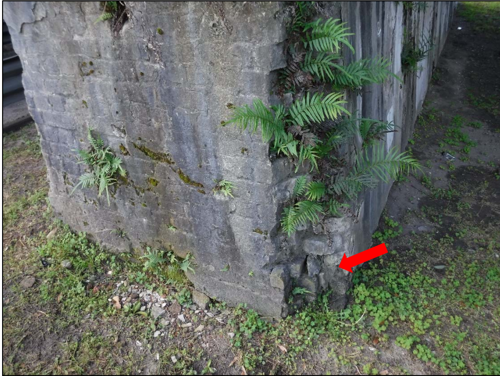
Photograph 35 – Missing Brick at Pier 2
