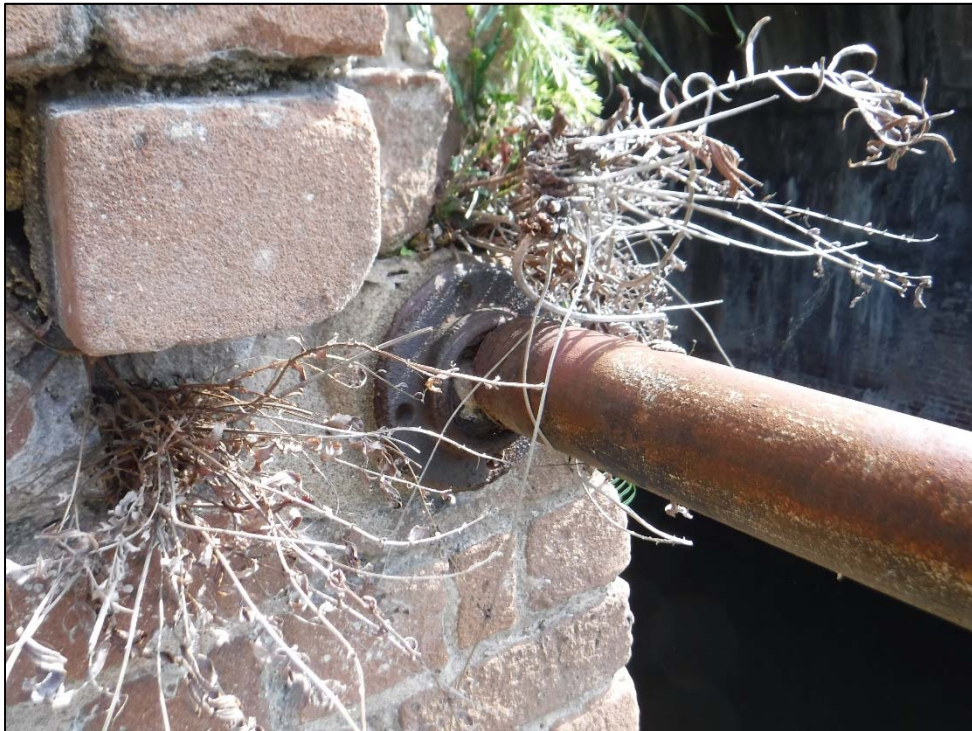
Photograph 66 – Disconnected Guardrail at Arch 1
