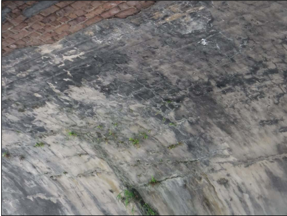
Photograph 85 – Map Cracking in Mortar in Arch 3
