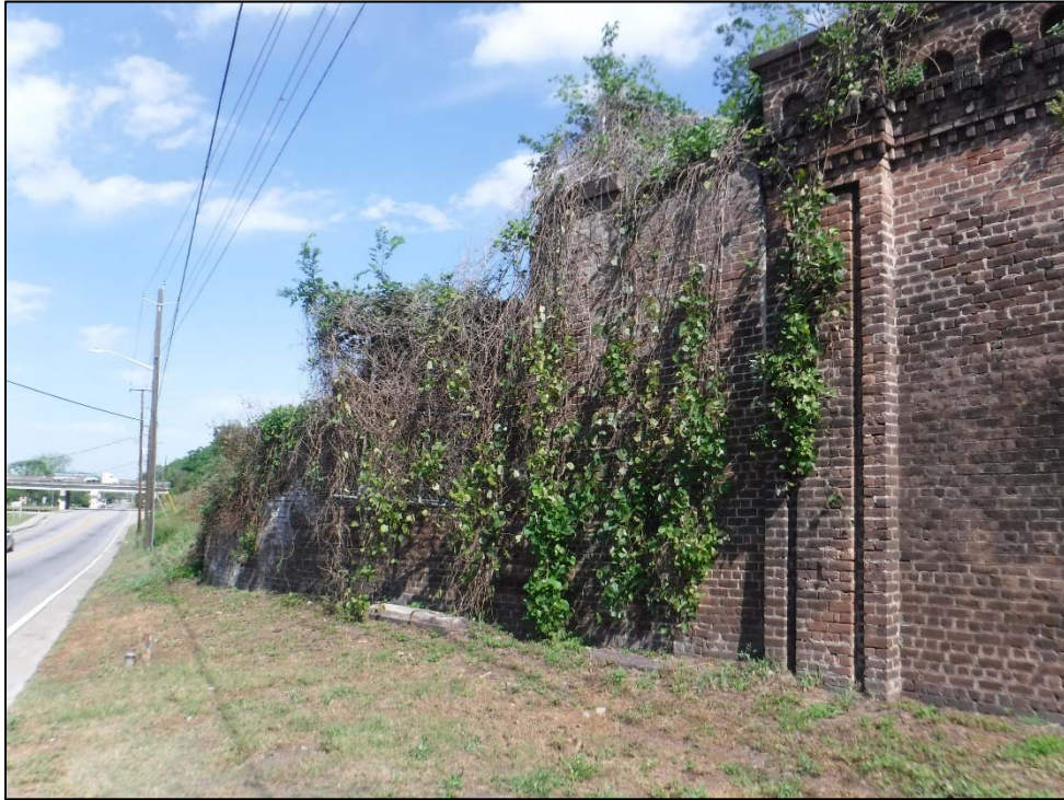
Photograph 101 – Vegetation Growth on Southwest Wingwall
