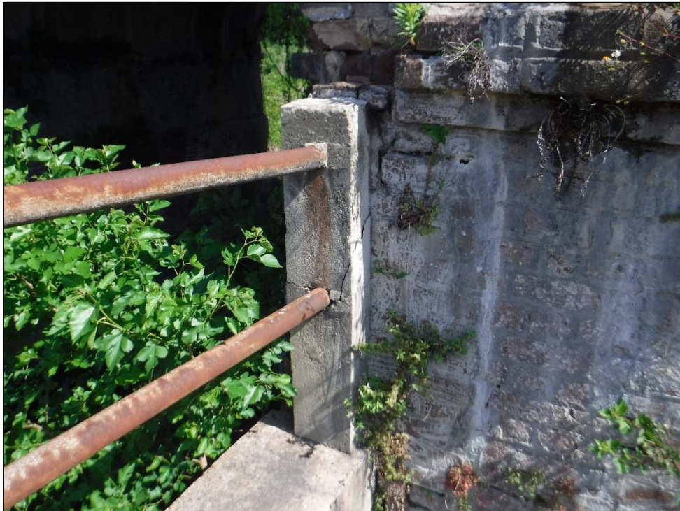
Photograph 68 – Cracking Near Rail Connection at Arch 1
