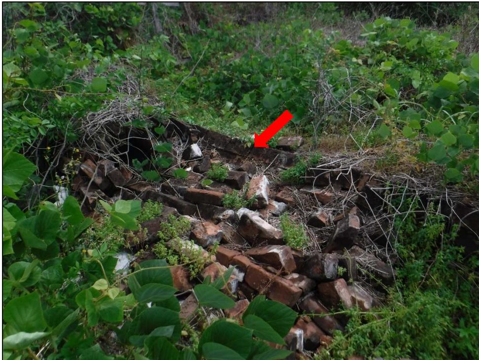
Photograph 16 – Collapsed Portions of Open Drainage Arches
