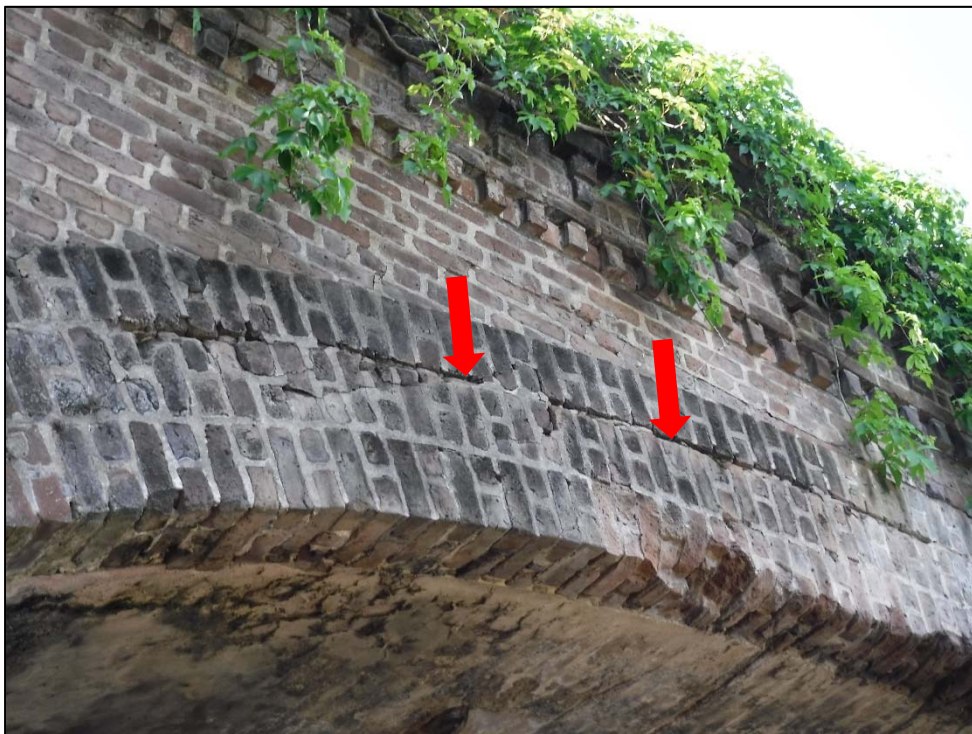
Photograph 30 – Damaged Mortar Joint at Arch Ring at Arch 3
