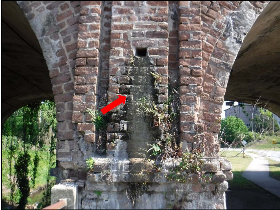
Photograph 59 – Weep Hole with Staining at Pier 1
