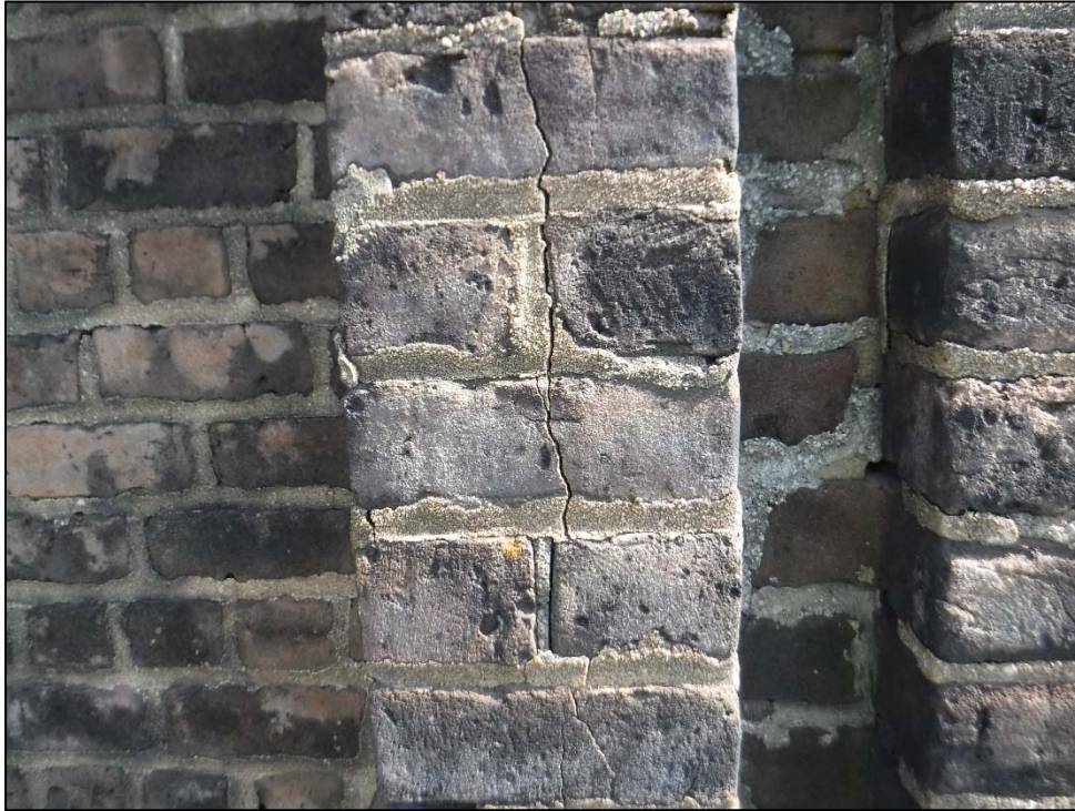
Photograph 49 – Crack with Damaged Bricks
