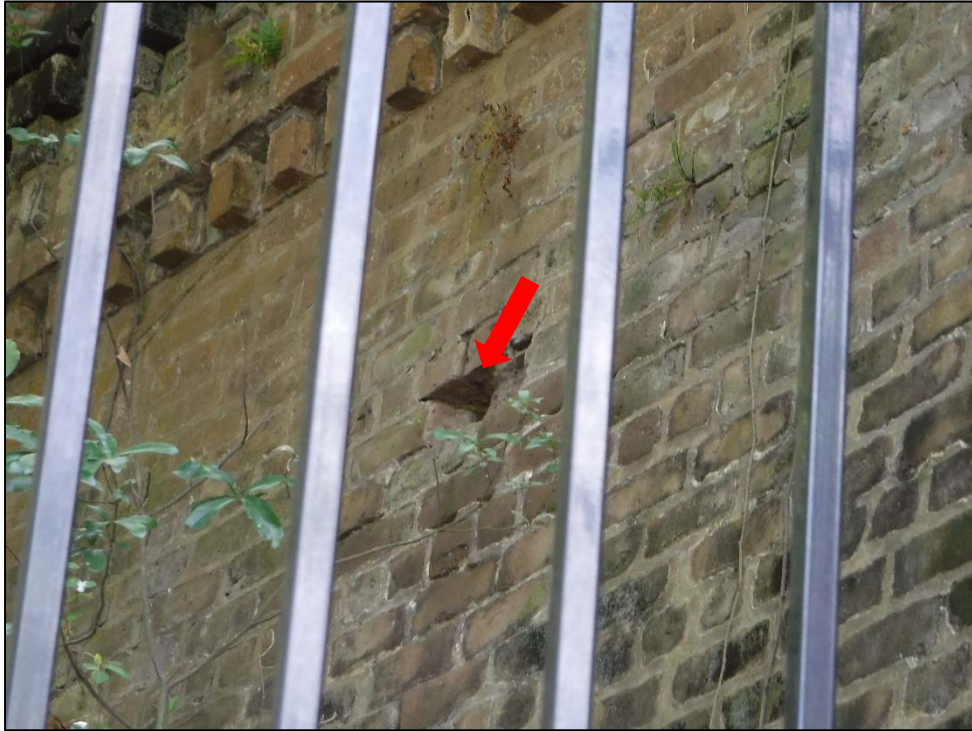
Photograph 39 – Broken Brick in Arch 4
