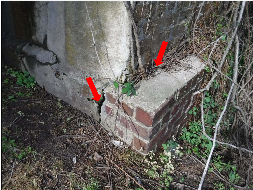
Photograph 26 – Separation and Displaced Brick with Vegetation at Pier 1
