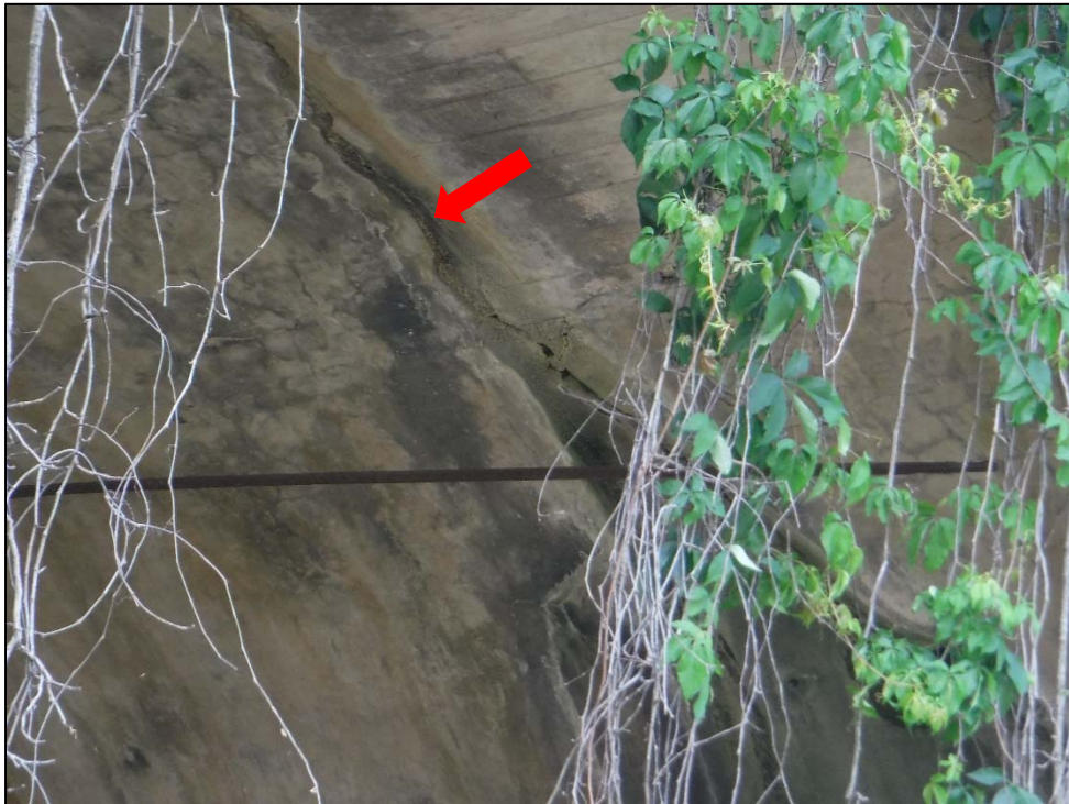
Photograph 72 – Crack with Spalled Mortar in Arch 1
