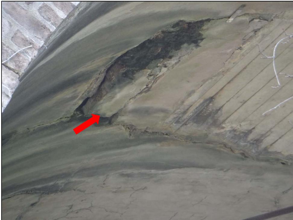
Photograph 74 – Crack with Spalled Mortar in Arch 1
