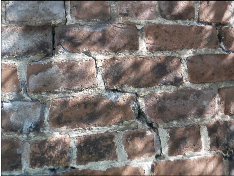
Photograph 93 – Diagonal Crack with Damaged Brick in Southwest Wingwall
