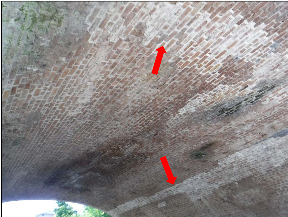
Photograph 88 – Evidence of Previous Repairs to Brick and Mortar Joints in Arch 4
