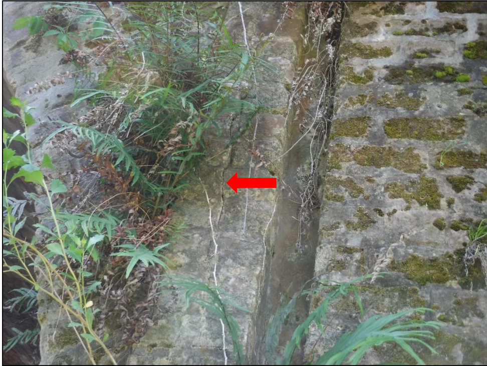
Photograph 29 – Crack with Damaged Bricks at Pier 2
