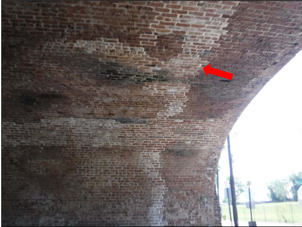
Photograph 89 – Evidence of Previous Repairs to Brick and Mortar Joints in Arch 4
