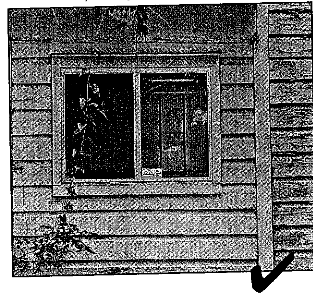
Siding should be applied in a horizontal fashion, with overlapping boards or weatherboard, as pictured above. Also, it is best to approximate the width of wood siding used traditionally in Cuyler-Brownsville.
