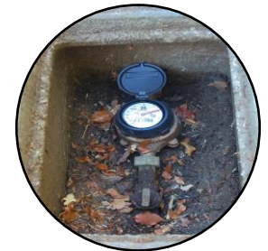
Water Meter Leaks
